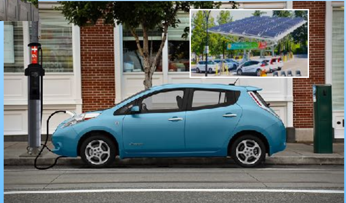
ELECTRIC VEHICLE CHARGING
