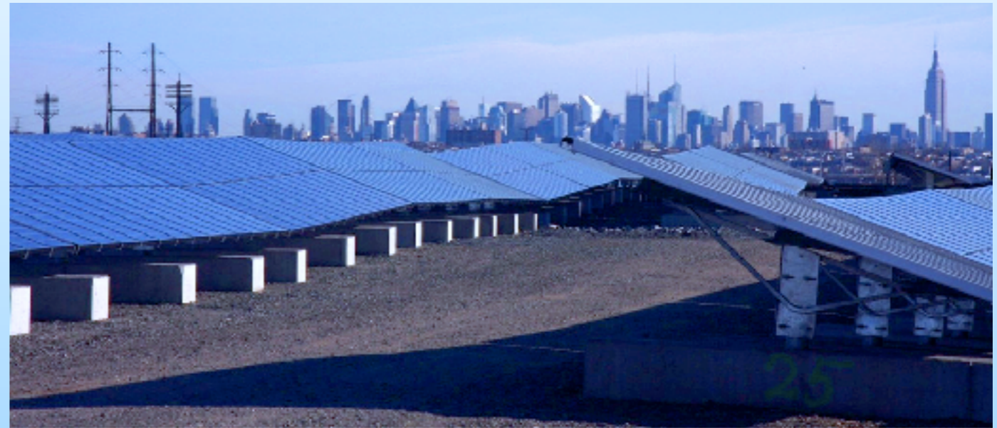
A solar installation on a capped landfill in New Jersey.
