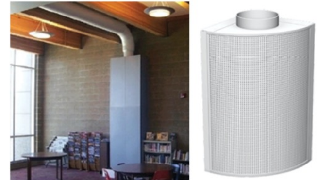
Figure 34 Side wall mounted displacement ventilation.
