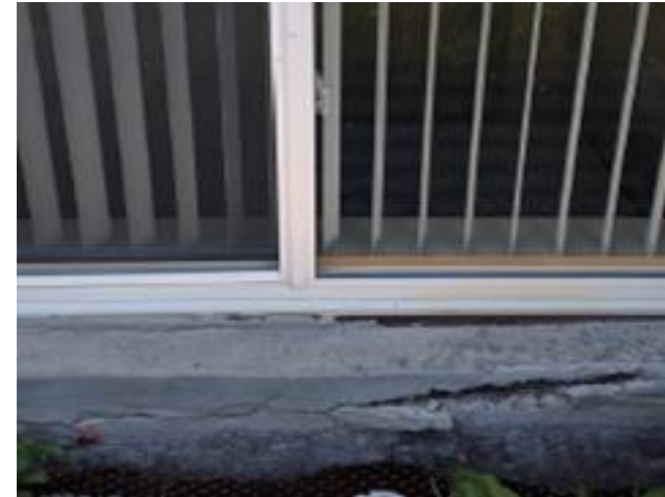
Cracking at Windows
