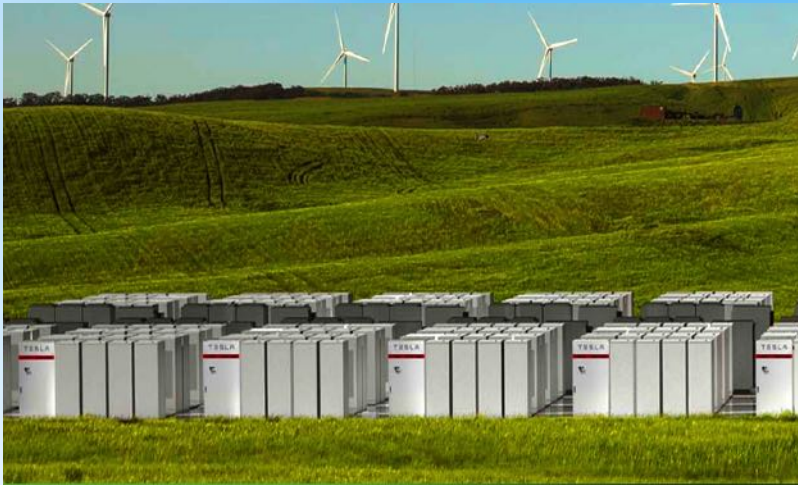
HORNSDALE POWER RESERVE SOUTH AUSTRALIA
