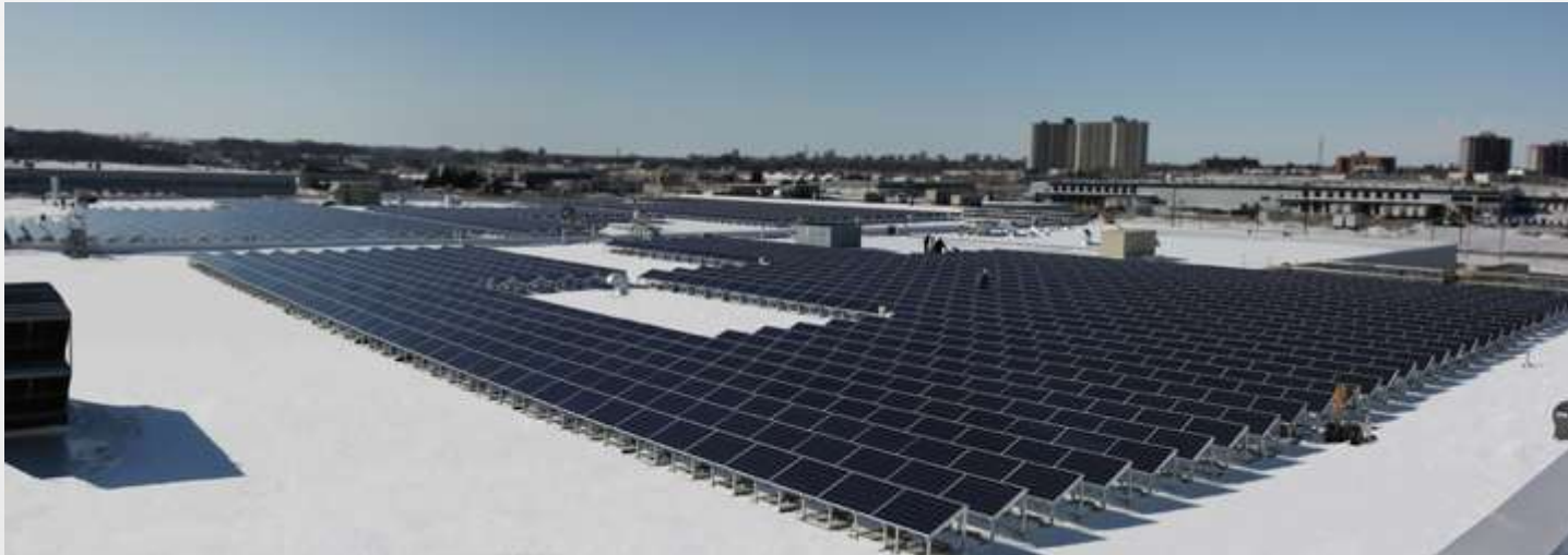
Kitchener Operations Facility – solar roof
