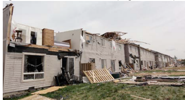
Figure B2: Structural roof failures (Angus, ON 2014)
