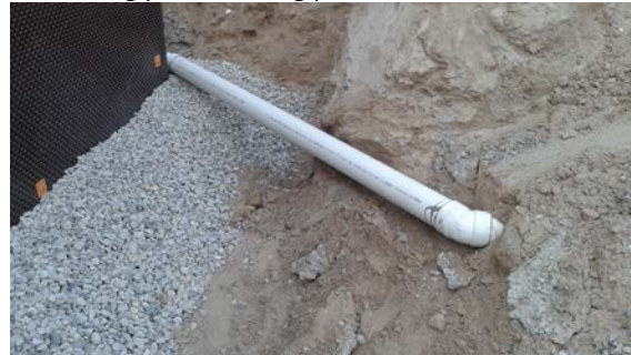
Figure A5: Newly installed building sewer (storm) illustrating poor bedding practices
