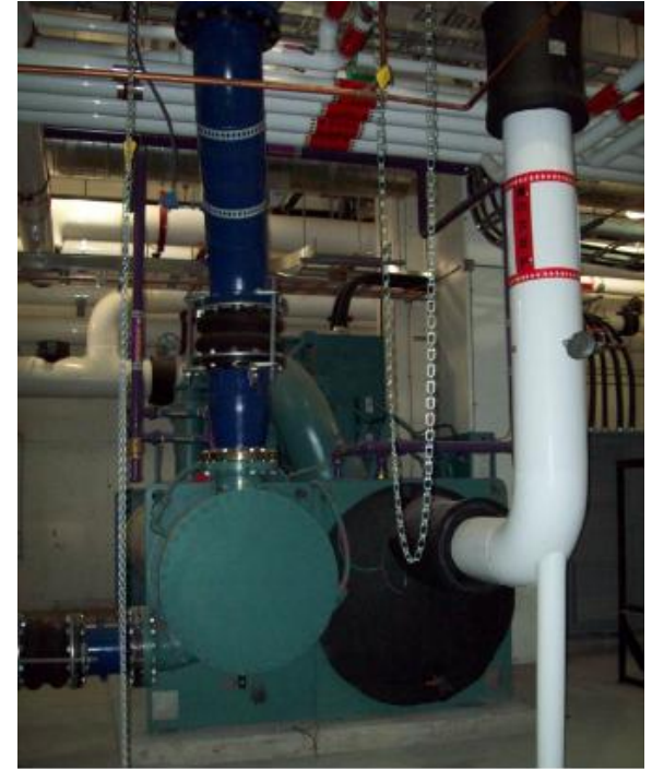
Regent Park Central Energy Plant Chiller Level. (Source: RPEI)
