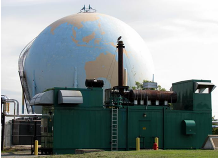
Woodward Wastewater Treatment Plant BioGas Storage in Globe
