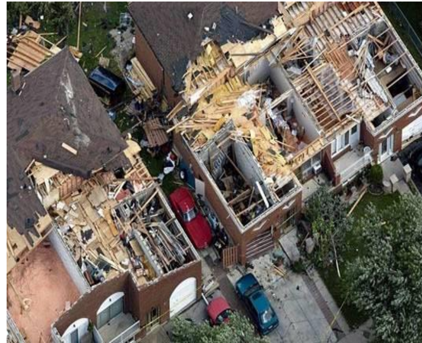
Photo: Tornado damage in Vaughan, 2009
